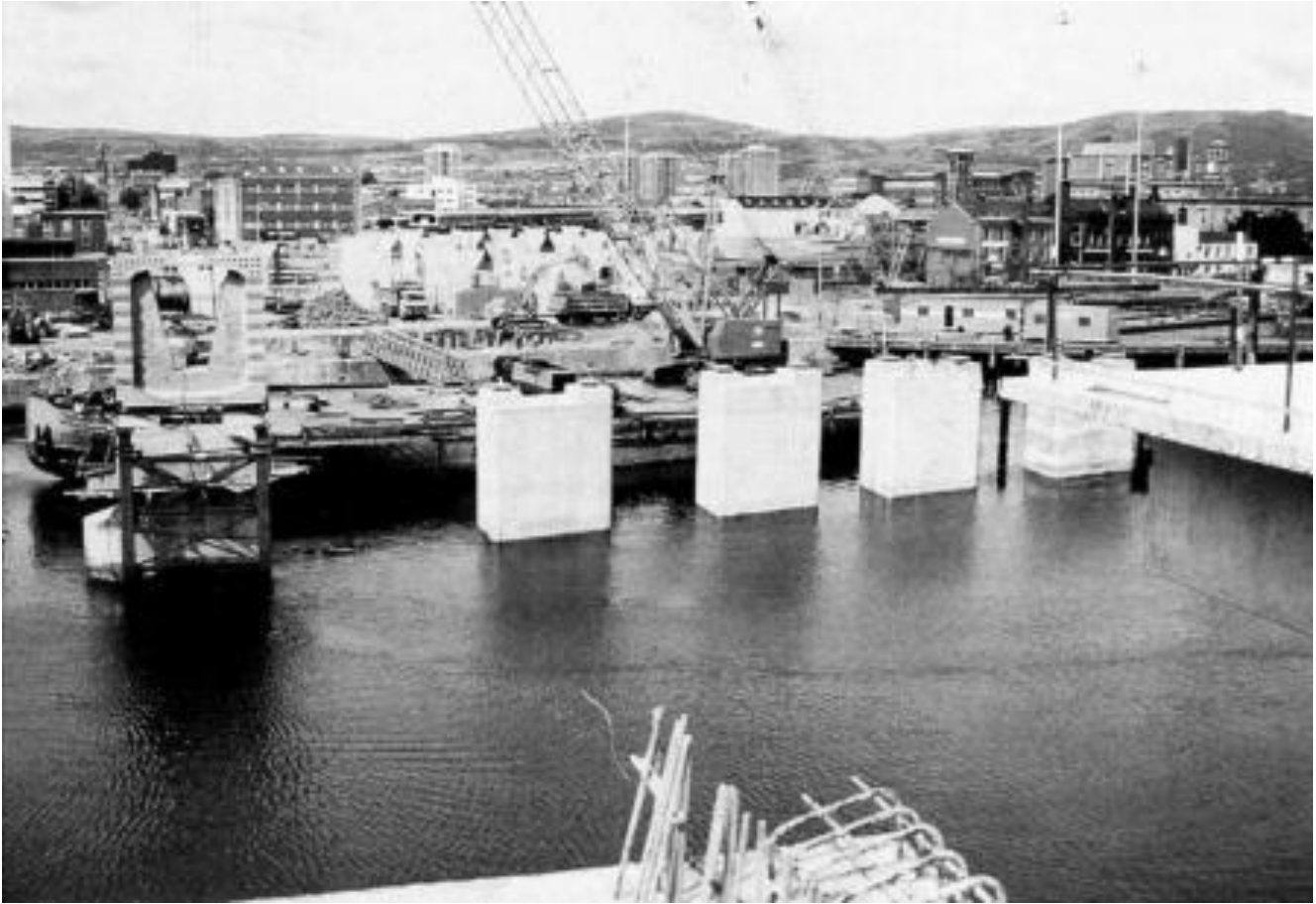
Looking towards Donegall Quay from the east bank of the Lagan on 17 th August 1993. On the left, work on the railway bridge is forging ahead while the piers for the road bridge are seen on the right. (D. Grimshaw)
